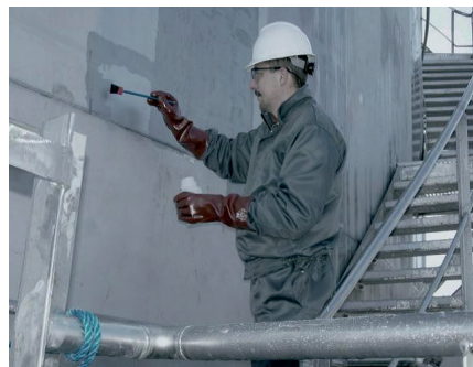
Photo: Site pickling with Gel 122, easy to apply thanks to its free flowing consistency
